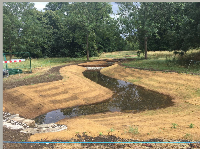
Natural drainage system at the Swale
